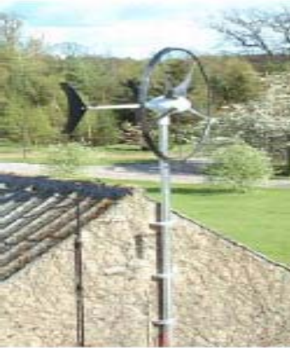
Gable mounted wind turbine (source Entec)
