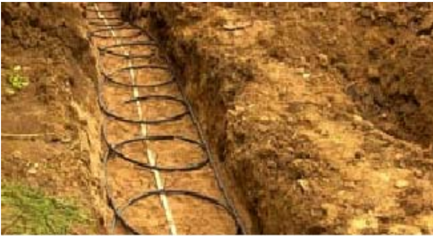
Ground source heat pump GSHP- ground loop in trench system (source DTI website- Entec)
