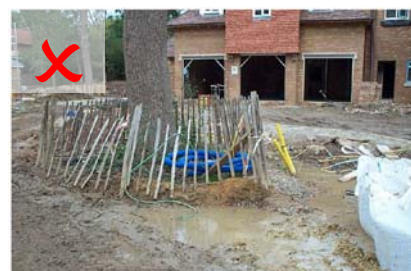
Picture 1: Non-compliant tree protective fencing – it is too close to the tree and is not strong enough to withstand impacts. The result being that the ground area around the tree has suffered from compaction and waterlogging, which will ultimately result in decline or death of the tree.
